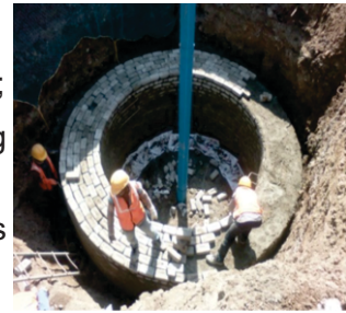
RWH System at MIHAN Depot
