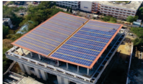
Solar Panels at Metro Bhawan
