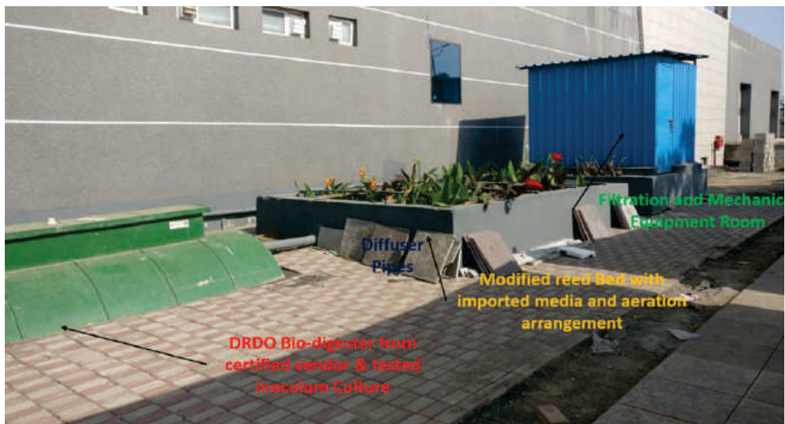
Actual Picture of Bio-digester installation at Metro Station
