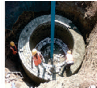
RWH System at Mihan depot
