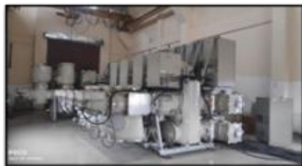
132kV GIS installed at Range Hill RSS
