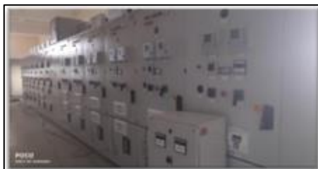
25kV GIS board installed at Range Hill RSS
