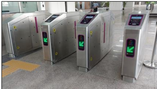
AFC gates installed at Sant Tukaram Nagar Station, Pune
