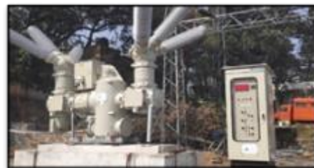
132kV Hybrid GIS installed at Ganeshkhind grid Substation
