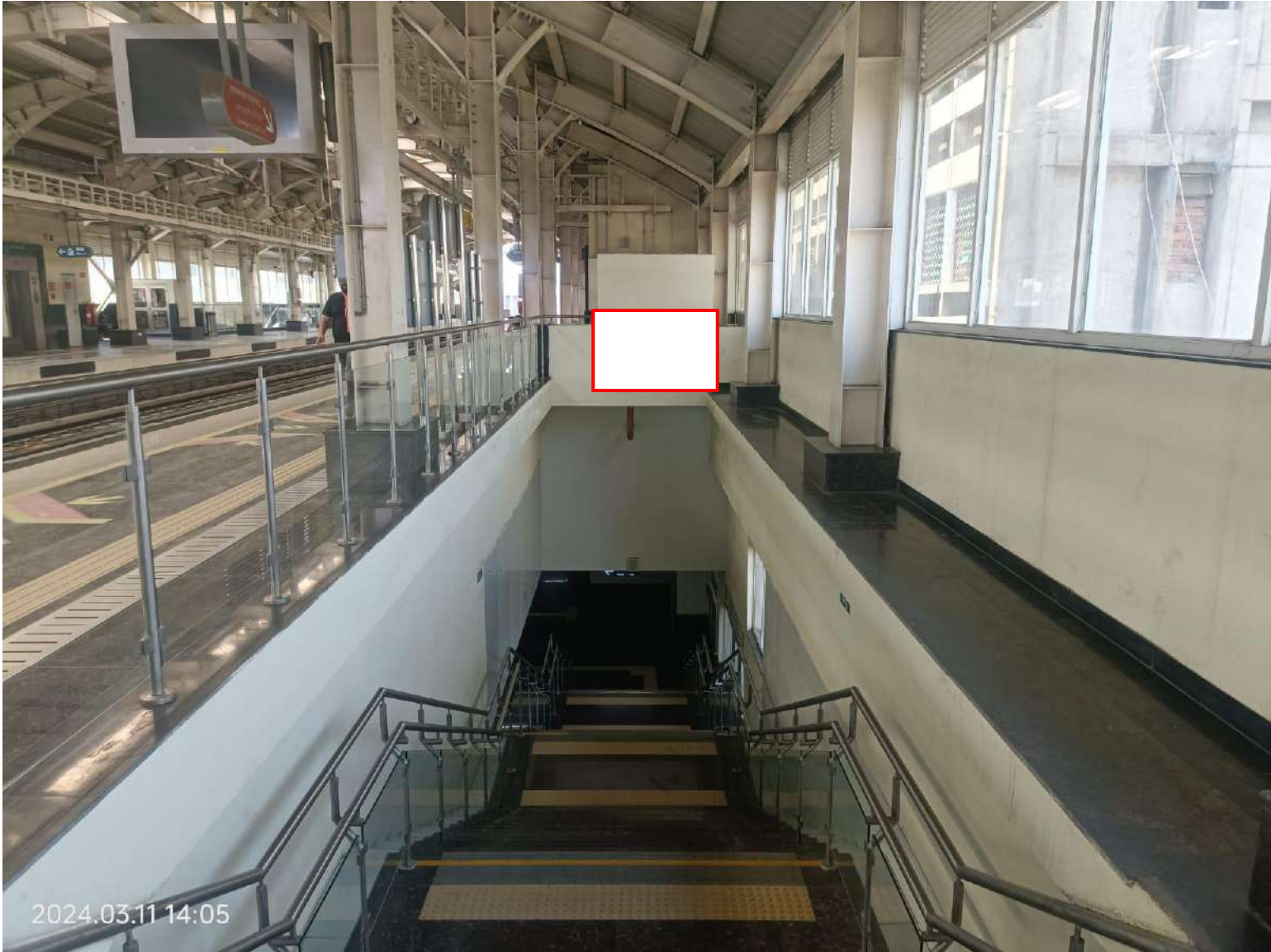
Dosar bhawan metro station platform 2 staircase upper Wall 8x5
